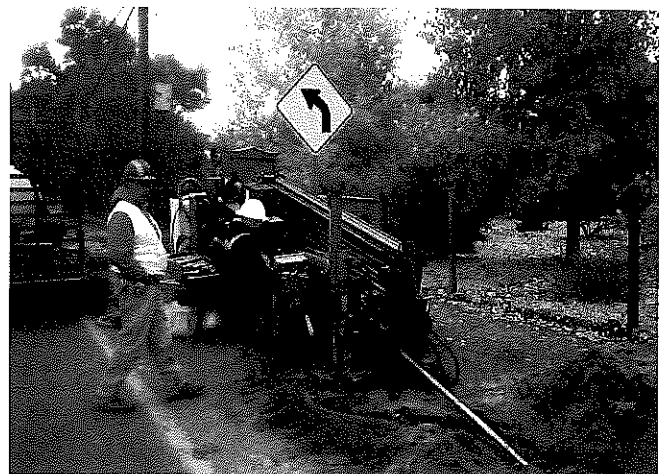
Directional drilling was used to "surgically" install the septic-tank effluent-pump collection pipe between existing utilities in the narrow right-of-way. Souder, Miller & Associates
